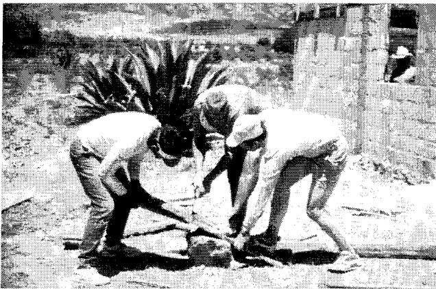
Fig. 5. Mexican, Russian and American workers cut formwork for the HfH house under construction behind them.
